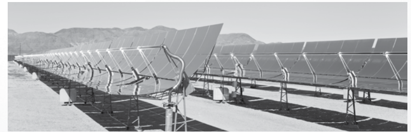
Fig. 3.3.1 Solar field of a concentrated solar power plant
